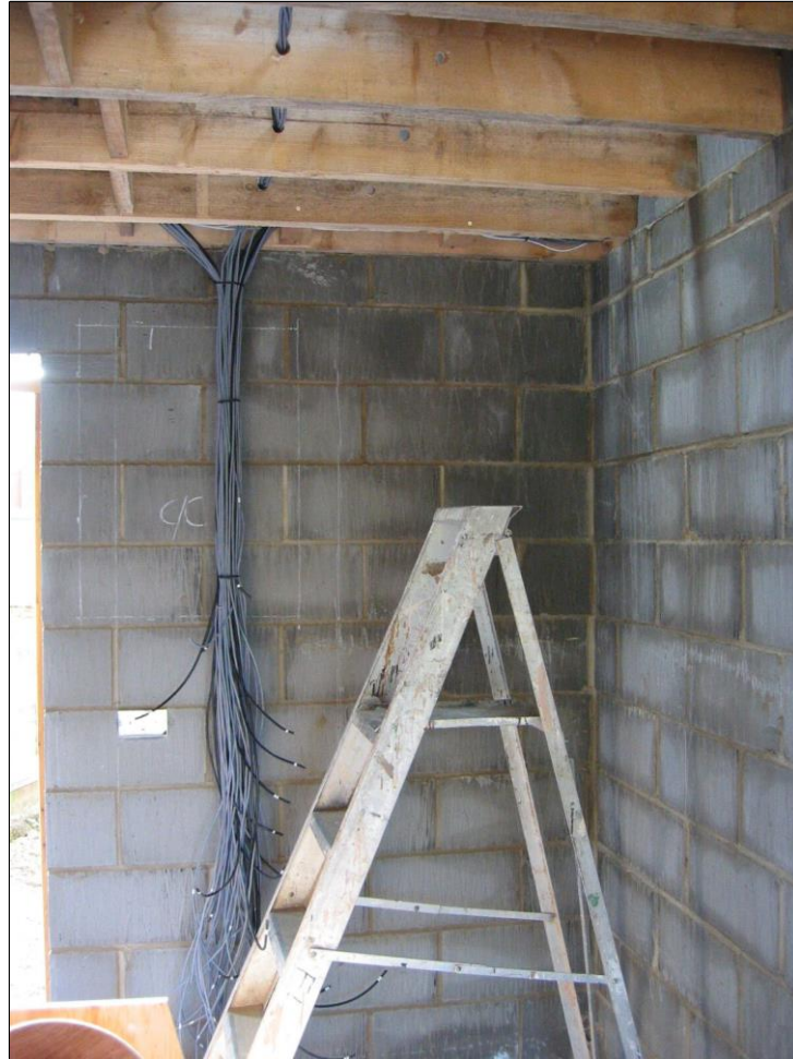
Cabling at the data cabinet location in garage
