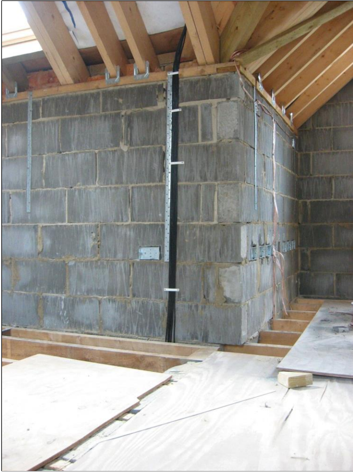
Cabling feeding from garage up to roof space
